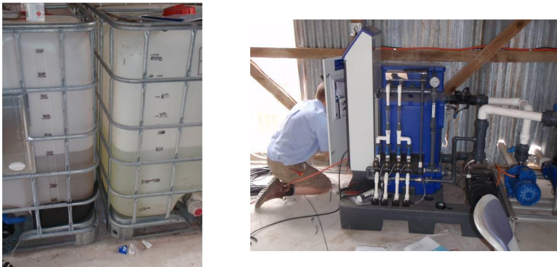
Figure 12 ‘A’ and ‘B’ tanks of concentrated nutrient solution (left) and fertigation unit (right)
